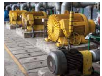
Only a few parameters are required to set up the motor and the protective functions.
